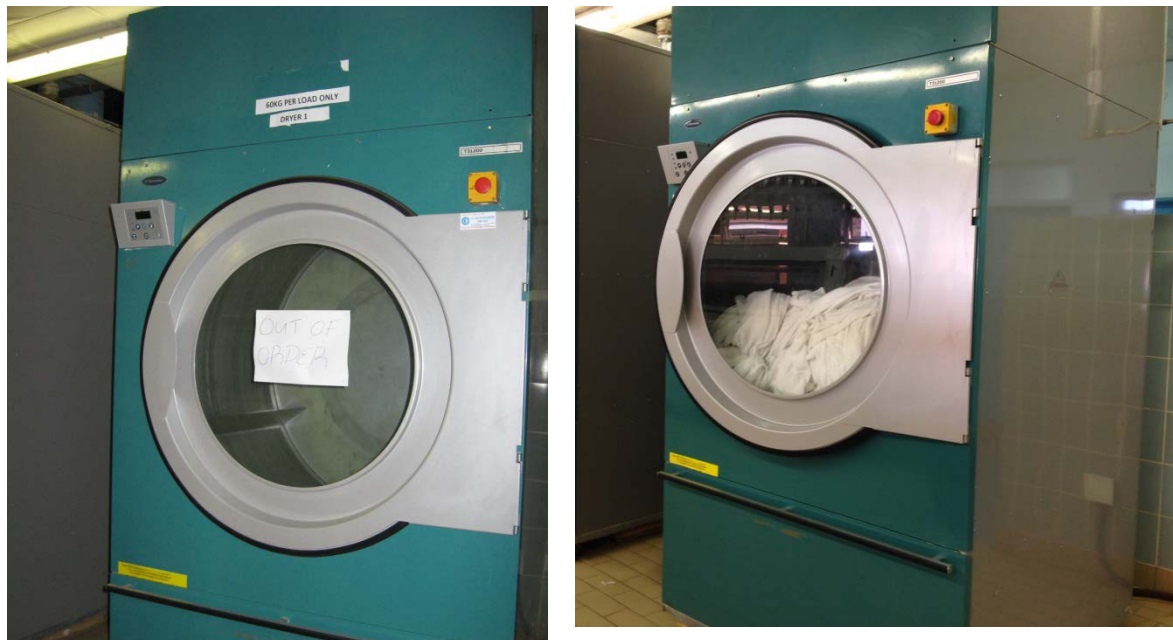
Figure 4: Washing machines that were broken before outsourcing are now in working order
